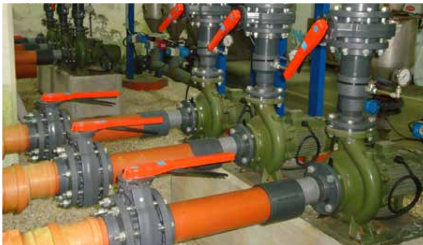
NR. 25 IR4P 65-250NB SPAIN PVC PRODUCTION PLANT
