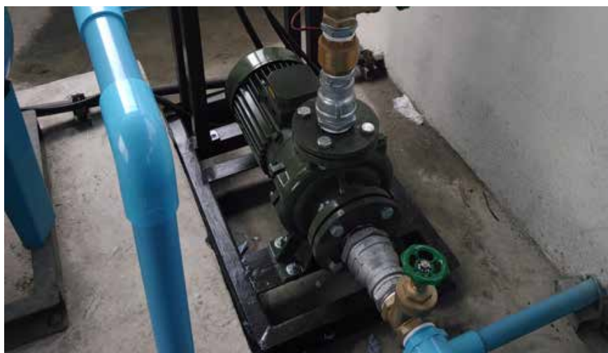
NR. 1 IR 50-160B THAILAND WATER SUPPLY IN A HOTEL
